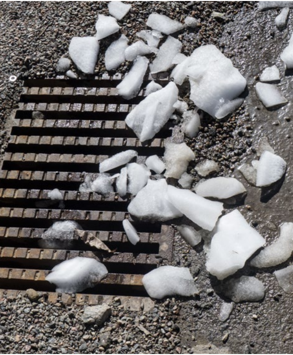
A surface water drain is designed to drain stormwater away from impervious surfaces such as streets, parking lots, sidewalks and dikes. Photo: Swedish EPA
